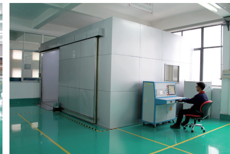
Fully shielded partial discharge pressure test equipment
